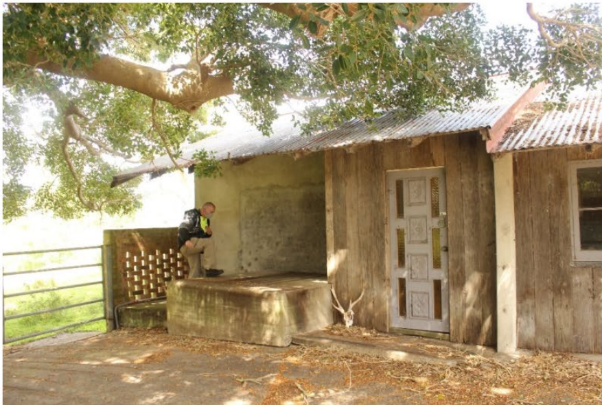
Figure 12: Southern end of dairy building, showing raised milk storage area and recent vertical slab cladding (recycled bull pen fencing) and residential door which were added to the building during the 1990's modifications.
